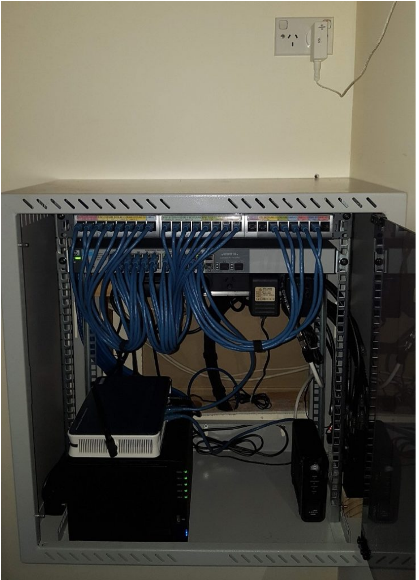
Photo 3: The whole cabinet. Note the small hole in the plaster above where the old power cable emerged.
